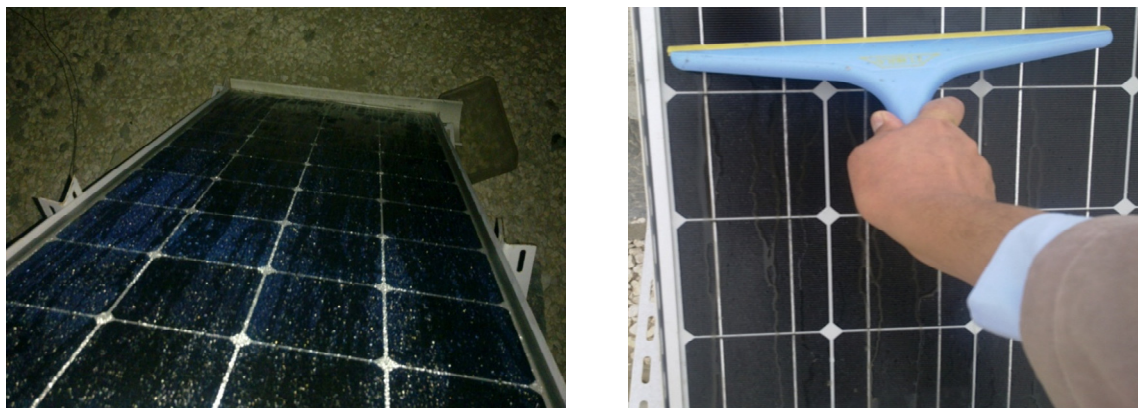
Figure 4: Dew condensation on the PV module surface (left) and scraping dew (right).
